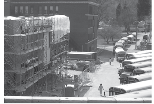
Looking down from the top of the retaining wall, façade work has begun at the elementary school building addition.
